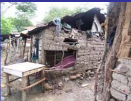
Rain damage at the Laurels
